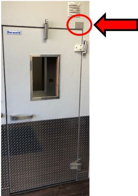
Picture 1.1. Arctic West Door; see location of the j-box where the heater cable is connected.
